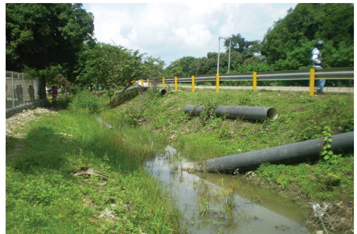
Despite the purchase of costly pipes, many pipes are incomplete and waiting by the roadside to be installed.
